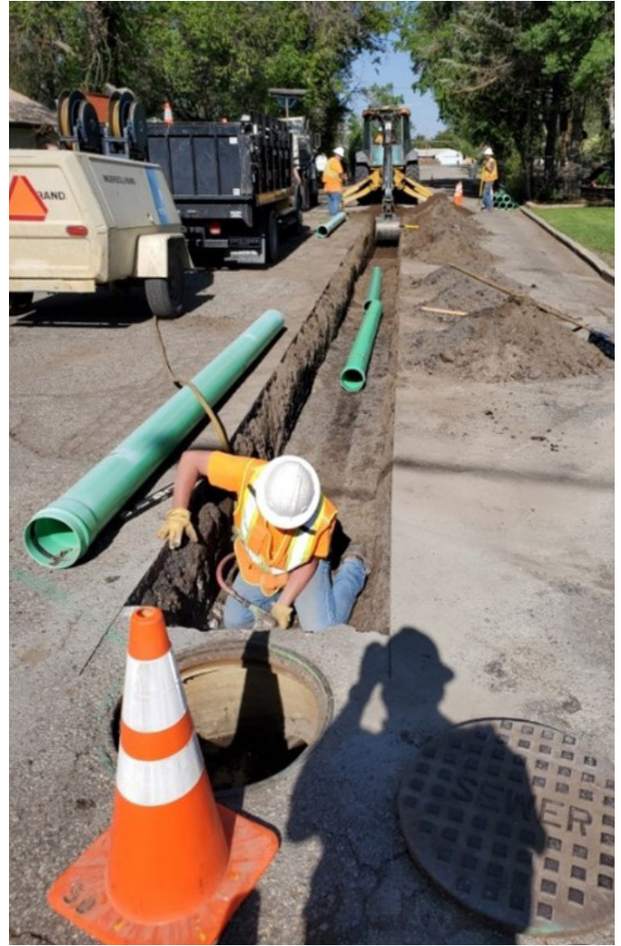
Installation of new water distribution infrastructure for the City of Alamosa (photo courtesy of City of Alamosa).
