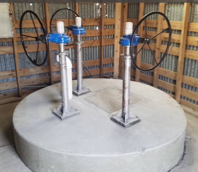
New reservoir outlet works for the Mountain Home Reservoir dam (photo by Wayne Schwab)
